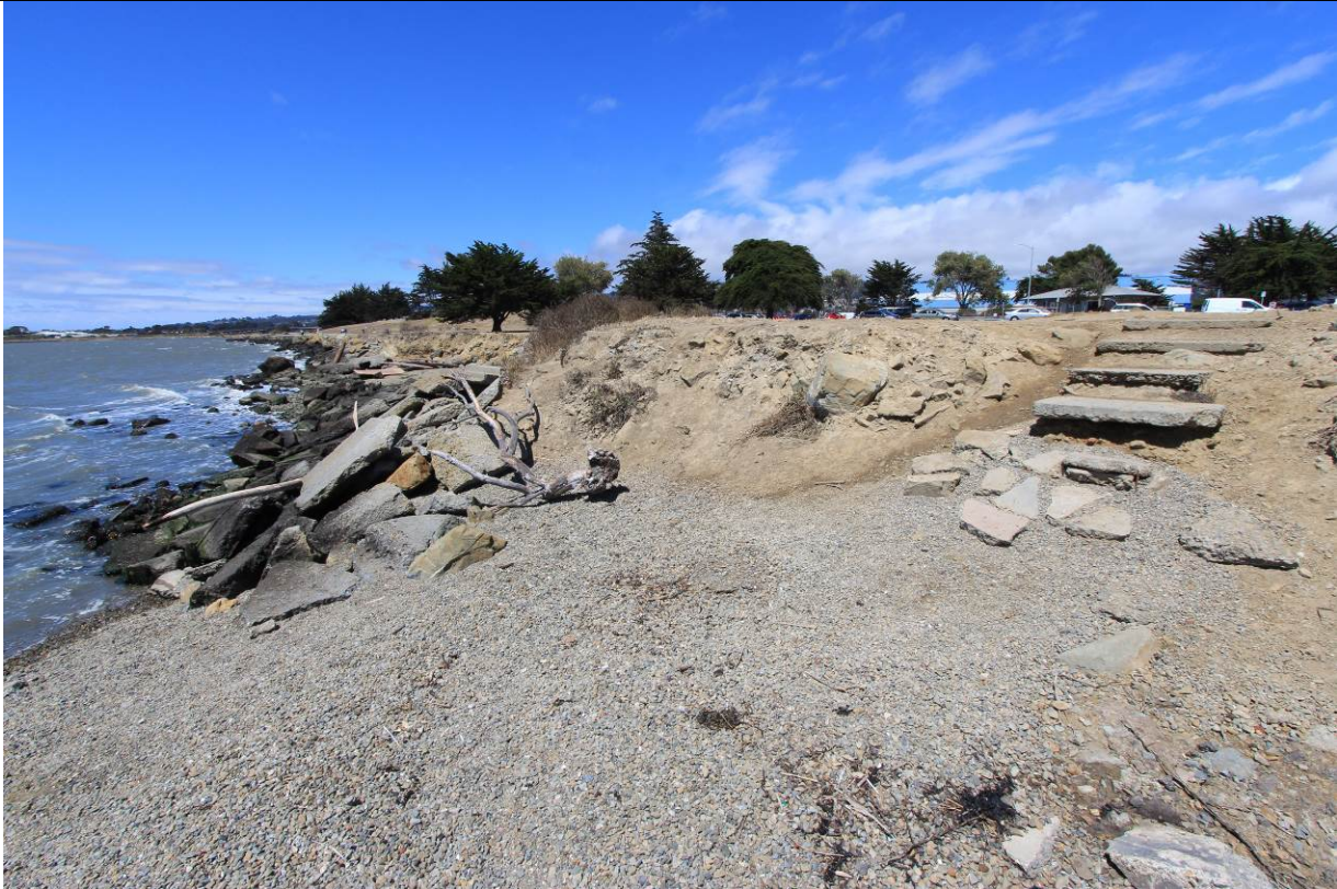
The existing launch is not accessible, with the eroded steps and submerged boulders making access challenging for all users. The District is in the process of engineering a new launch that will provide ADA access to the shore, which may feature an ADA ramp and a path of travel from the parking area and restrooms.
